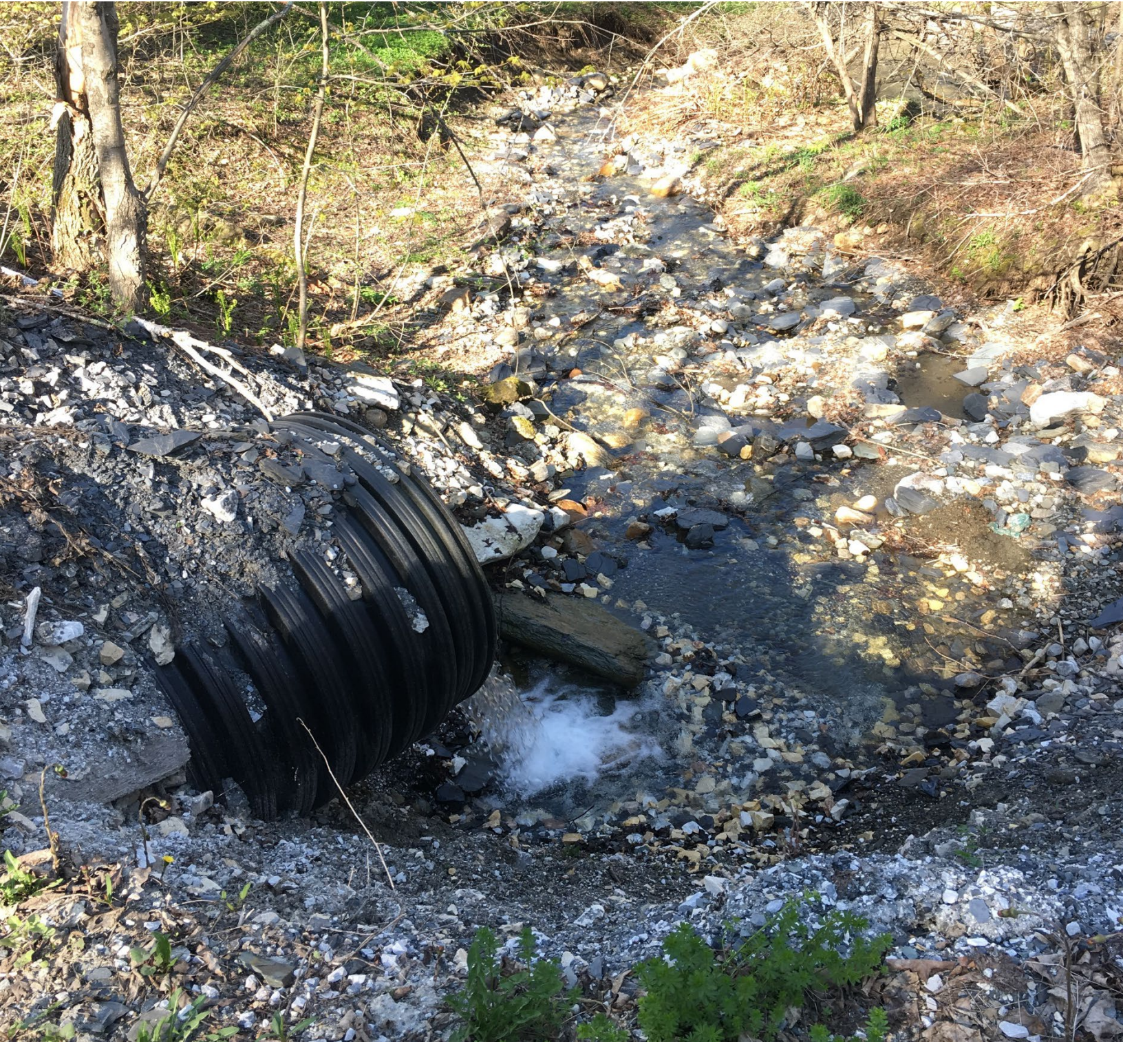
Little Village Road Culvert Washout - 2017
