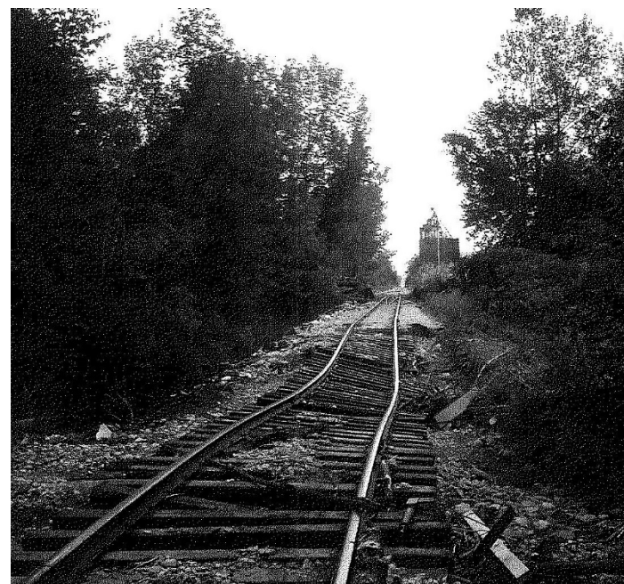
Railroad Track Damage from Tropical Storm Irene
